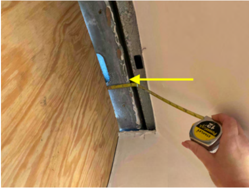
Photo 15 Unit No. 200 - View of existing framing 14G framing attached at concrete - Further investigation needed.
