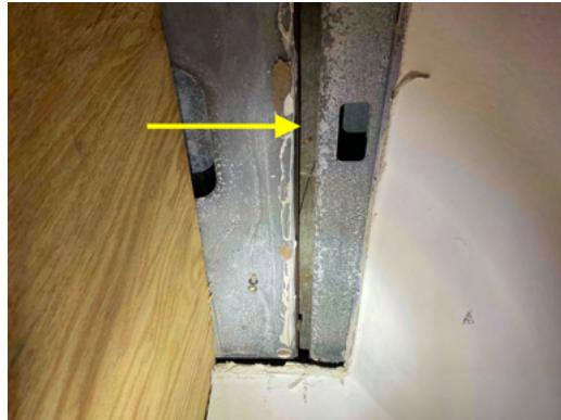
Photo 16 Unit No. 200 - View of existing framing 14G framing attached at ceiling - Further investigation needed.
