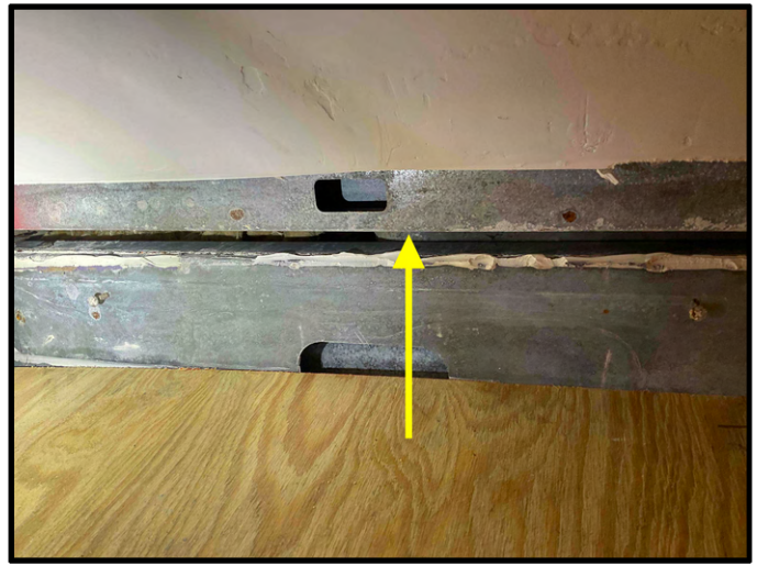
FIGURE 12 - Unit No. 200 - View of existing 14G framing attached at ceiling - Further Investigation Needed.
