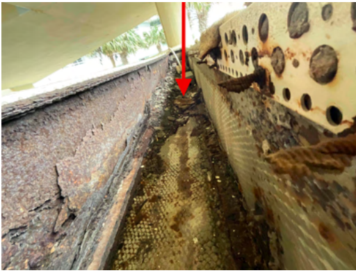
Photo 19 Porte Cochere - View of existing architectural beam with severely corroded framing.
