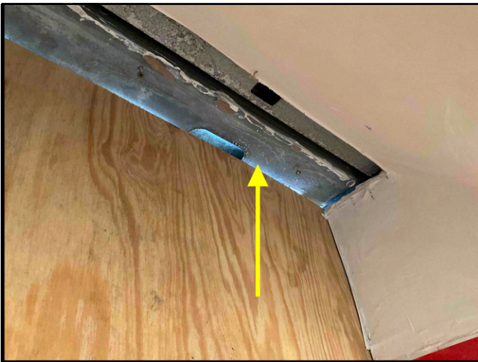
FIGURE 9 - Unit No. 200 - View of existing metal framing at head of window after existing window was removed - Work in Progress.
