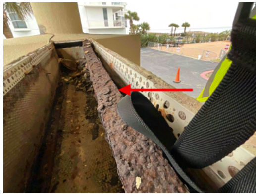
Photo 20 Porte Cochere - View of existing architectural beam with severely corroded framing.
