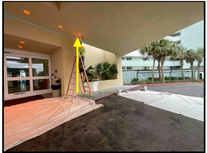
FIGURE 4 - Porte Cochere - View of crew members performing coating application at ceiling - Work in Progress.
