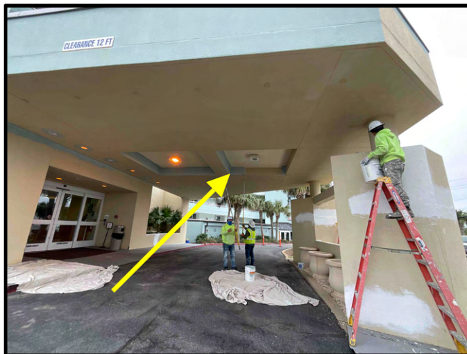
FIGURE 5 - Porte Cochere - View of crew members performing coating application at ceiling - Work in Progress.
