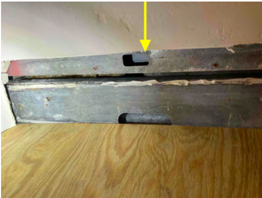
Photo 17 Unit No. 200 - View of existing framing 14G framing attached at ceiling - Further investigation needed.
