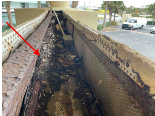
Photo 18 Porte Cochere - View of existing architectural beam with severely corroded framing.
