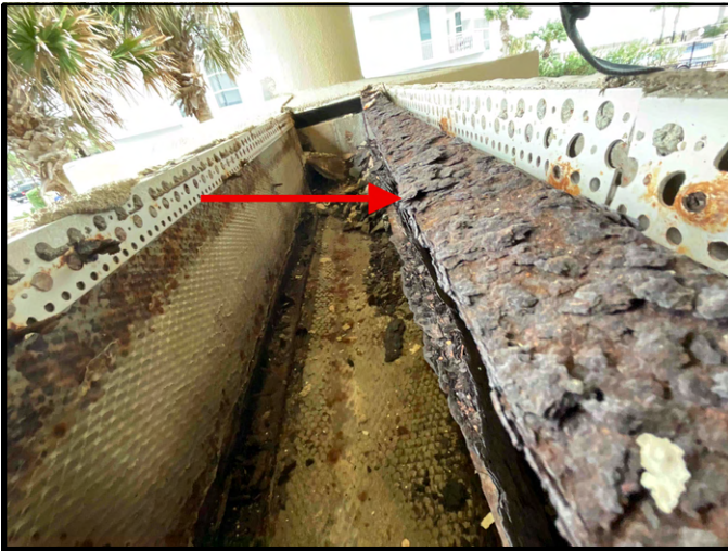
FIGURE 7 - Porte Cochere - View of existing architectural beam with severely corroded framing.
