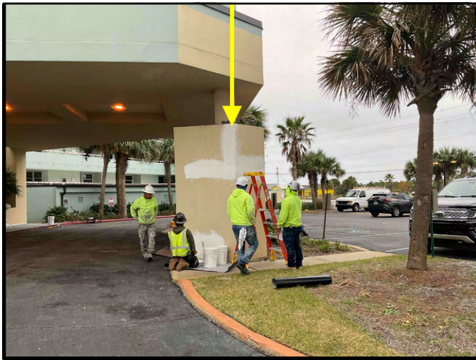
FIGURE 3 - Porte Cochere - View of crew members performing finish repairs at stucco column - Work in Progress.
