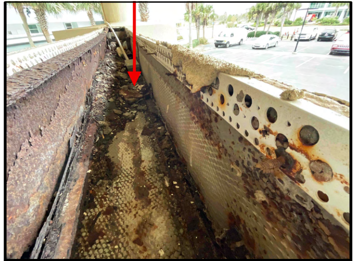
FIGURE 8 - Porte Cochere - View of existing architectural beam with severely corroded framing.
