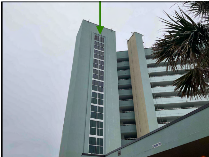
FIGURE 1 - View of new EFCO storefront windows installed at north elevation above Porte cochere.
