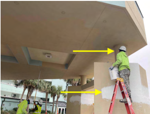
Photo 9 North Elevation - View of crew members performing finish repairs at stucco column and applying new coating at ceiling - Work in progress.
