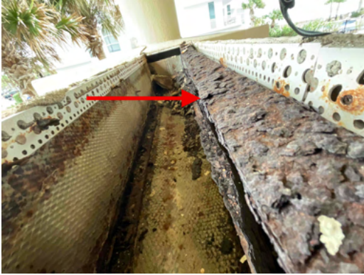
Photo 21 Porte Cochere - View of existing architectural beam with severely corroded framing.
