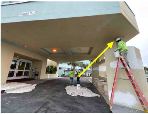
Photo 7 North Elevation - View of crew members performing coating application at ceiling - Work in progress.
