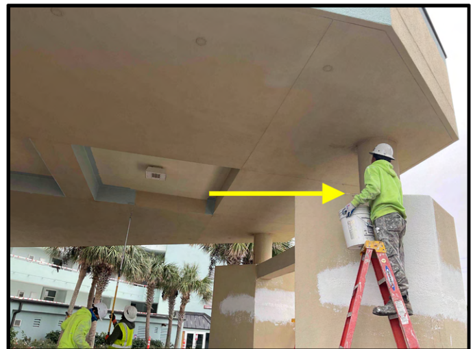
FIGURE 6 - Porte Cochere - View of crew members performing finish repairs at stucco column and applying new coating at ceiling - Work in Progress.
