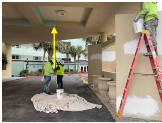
Photo 8 North Elevation - View of crew members performing coating application at ceiling - Work in progress.
