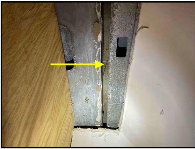
FIGURE 11 - Unit No. 200 - View of existing 14G framing attached to concrete - Further Investigation Needed.
