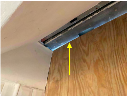
Photo 13 Unit No. 200 - View of existing metal framing at head of window after existing window was removed - Work in progress.
