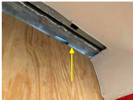
Photo 12 Unit No. 200 - View of existing metal framing at head of window after existing window was removed - Work in progress.
