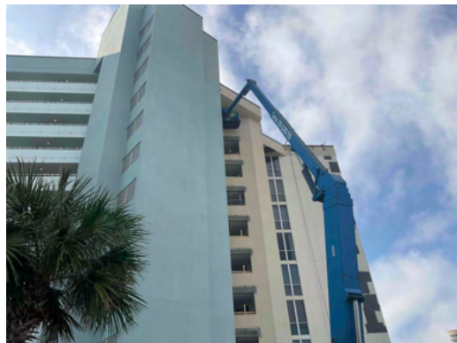
Photo 22 North Elevation - View of crew members applying new stucco at new header framing - Work in Progress.
