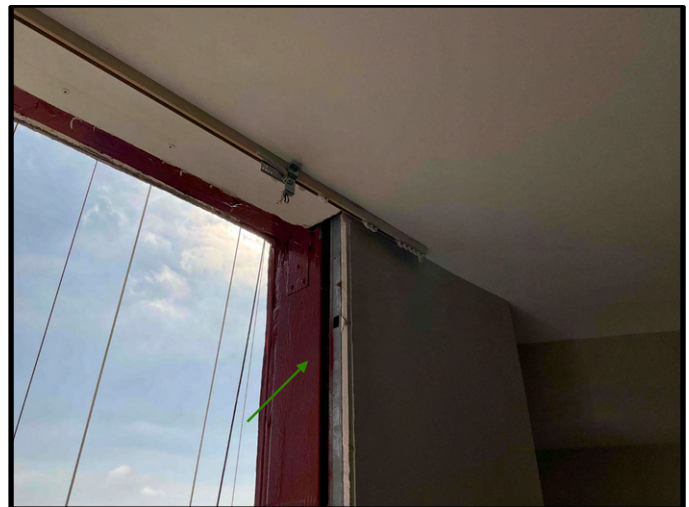
FIGURE 2 - Unit No. 200 - View of new FastFlash waterproofing installed at rough opening. Additional lumber to be installed at head of opening.
