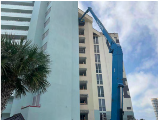
Photo 21 North Elevation - View of crew members applying new stucco at new header framing - Work in Progress.
