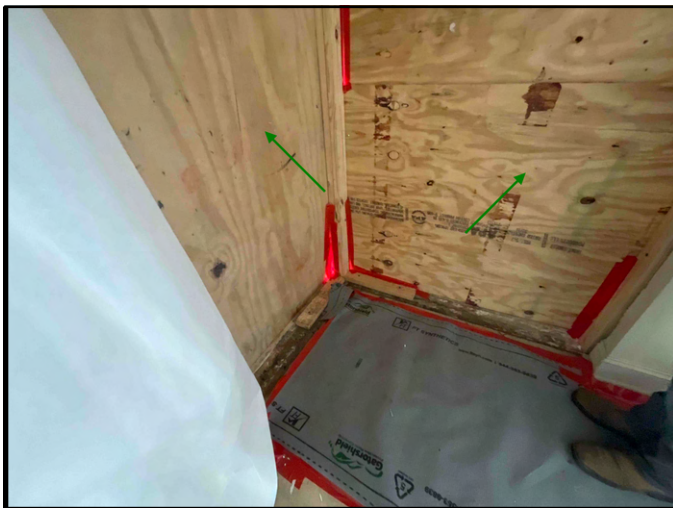
FIGURE 1 - Ground Floor Lobby - View of existing storefront window removed - Work in Progress.
