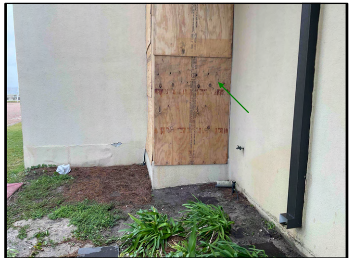
FIGURE 2 - Ground Floor Lobby - View of plywood installed at exterior side of existing storefront window removal - Work in Progress.
