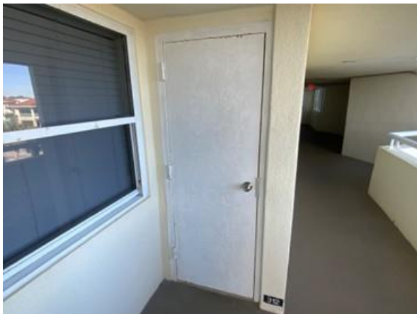
Photo 14 North Elevation – Common Walkway – View of minor corrosion at storage door.
