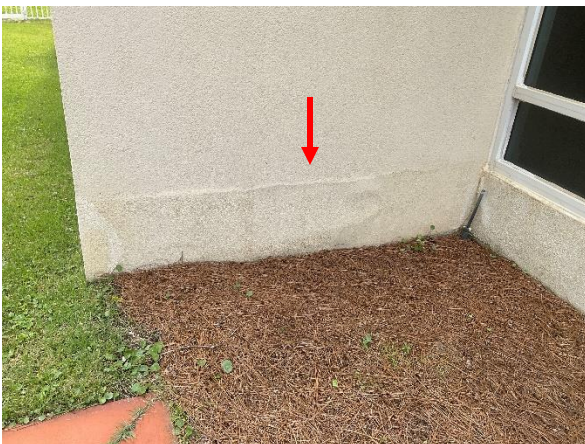
Photo 9 East Elevation – View of delaminated EIFS wall cladding – Isolated.
