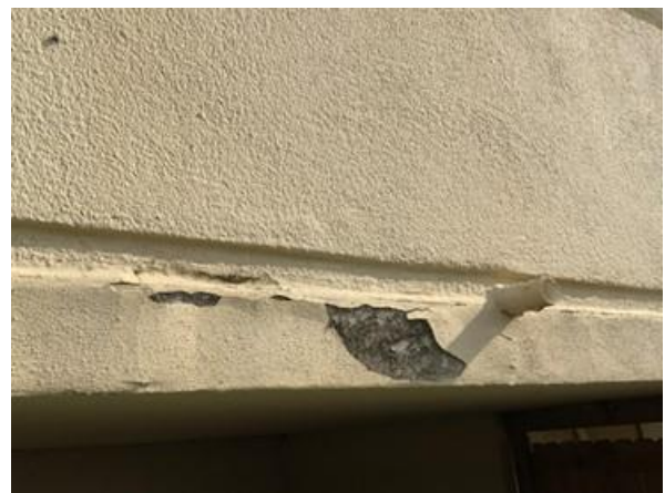
Photo 6 South Elevation – View of delaminated wall coating near balcony slab edge– Isolated.
