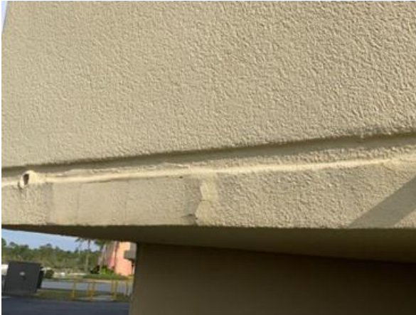
Photo 7 South Elevation – View of blistered wall coating near balcony slab edge– Isolated.
