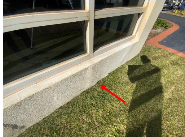
Photo 10 East Elevation – View of delaminated EIFS wall cladding – Isolated.
