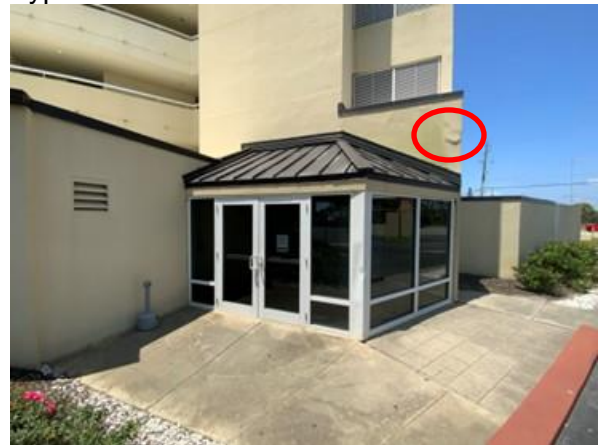
Photo 5 North Elevation – View of blistered wall coating – Isolated.
