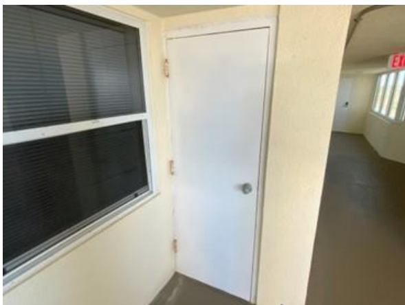
Photo 15 North Elevation – Common Walkway – View of minor corrosion at storage door.
