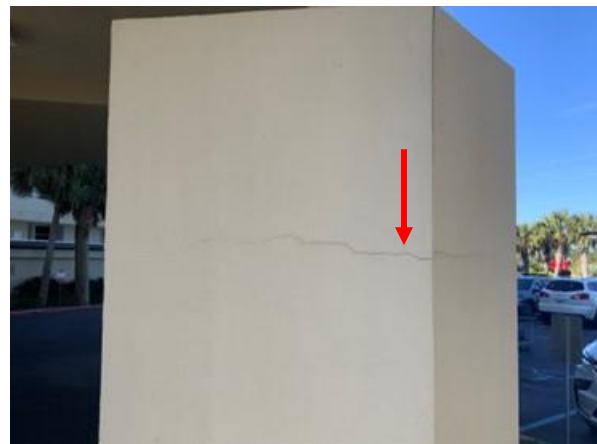
Photo 12 North Elevation - View of cracking in portecochere column – Isolated.
