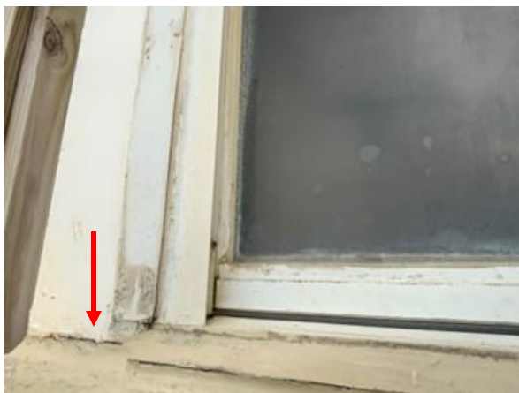
Photo 3 South Elevation – Overall view of windows, deteriorated sealants observed – Typical.
