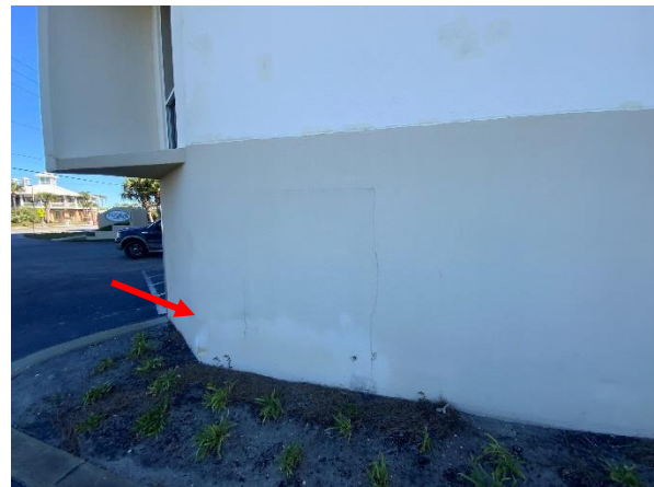
Photo 11 West Elevation - View of cracked and delaminated EIFS cladding – Isolated.
