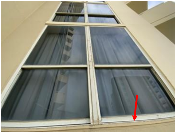
Photo 2 South Elevation – Overall view of windows, deteriorated sealants observed – Typical.
