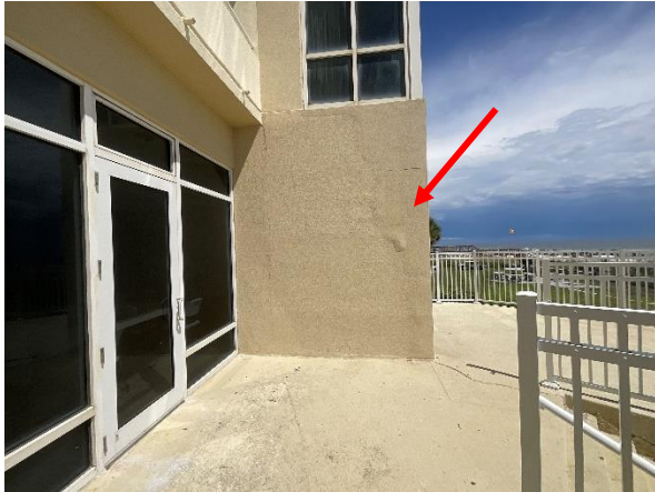
Photo 13 South Elevation - View of cracked and delaminated stucco cladding – Isolated.
