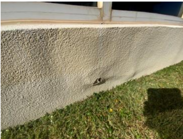
Photo 8 East Elevation – View of water damaged EIFS wall cladding – Isolated.
